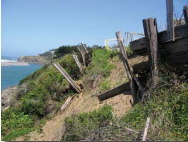
Failed retaining wall
