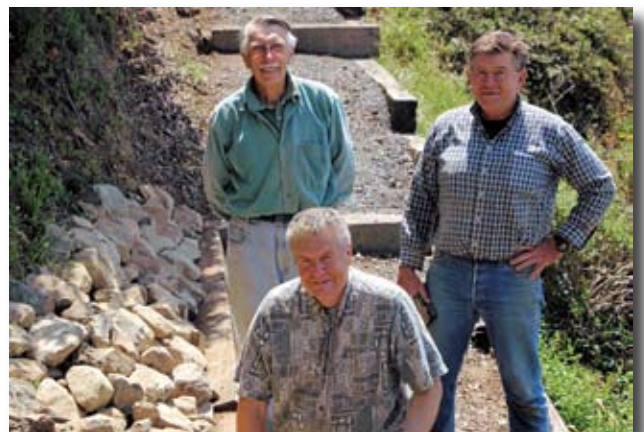
Ray Jackman (kneeling), Jim Suhr and John Petersen smile after finishing rock wall along the trail. Photo by Mary Sue Ittner
