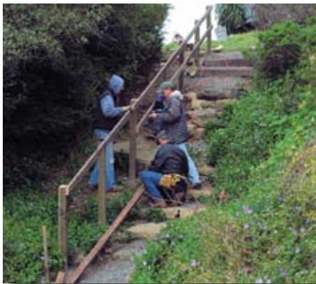
Bluff Trail volunteers put railing for steps into place. Photo by Mary Sue Ittner
